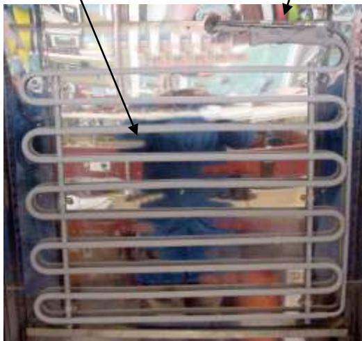
'Frosted' Evaporator & 'Frosted' Surge Pot compressor
