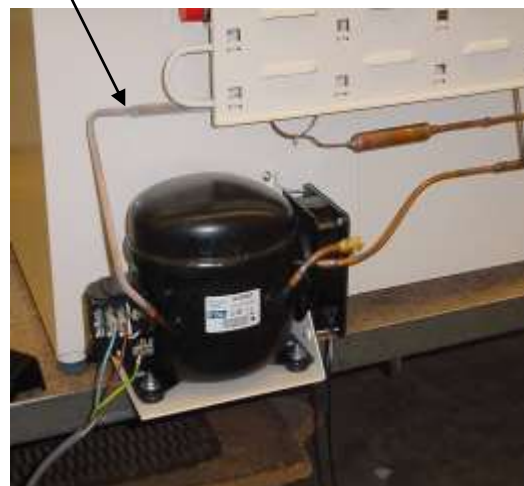
'Frost' on line to compressor
