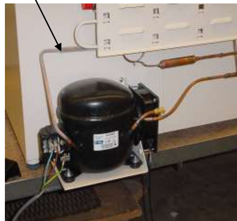
'Frost' on line to compressor
